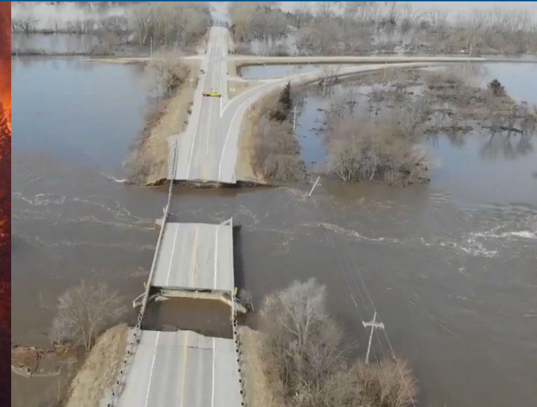
Nebraska flooding, 2019 Photo – CBS News
